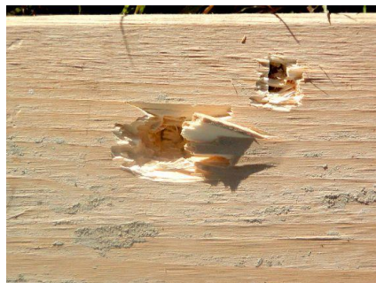
Figure 4. Entrance hole through a wooden board
